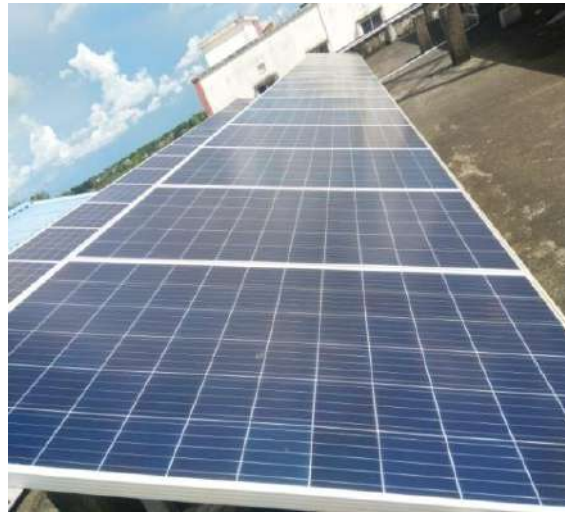
Solar Panel of 17Kw on Terrace of School
