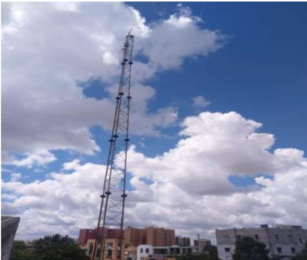
Lightening Arrestor of ASM
